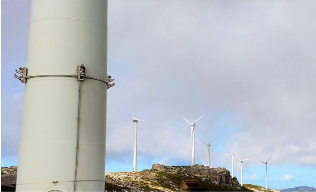
Figure 93: Installation of a Bird Monitoring System at the JWPPr Energy Wind Farm in Stavros Evia
